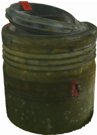
Damaged wellhead and repair section based on 3D model
